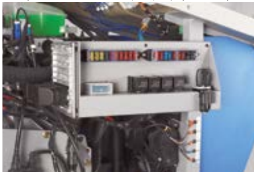
Relays, fuses, and an anti-start (PATS) employed in the system.
